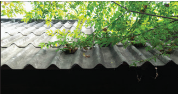
✗ Overgrown trees can cause roof damage.
